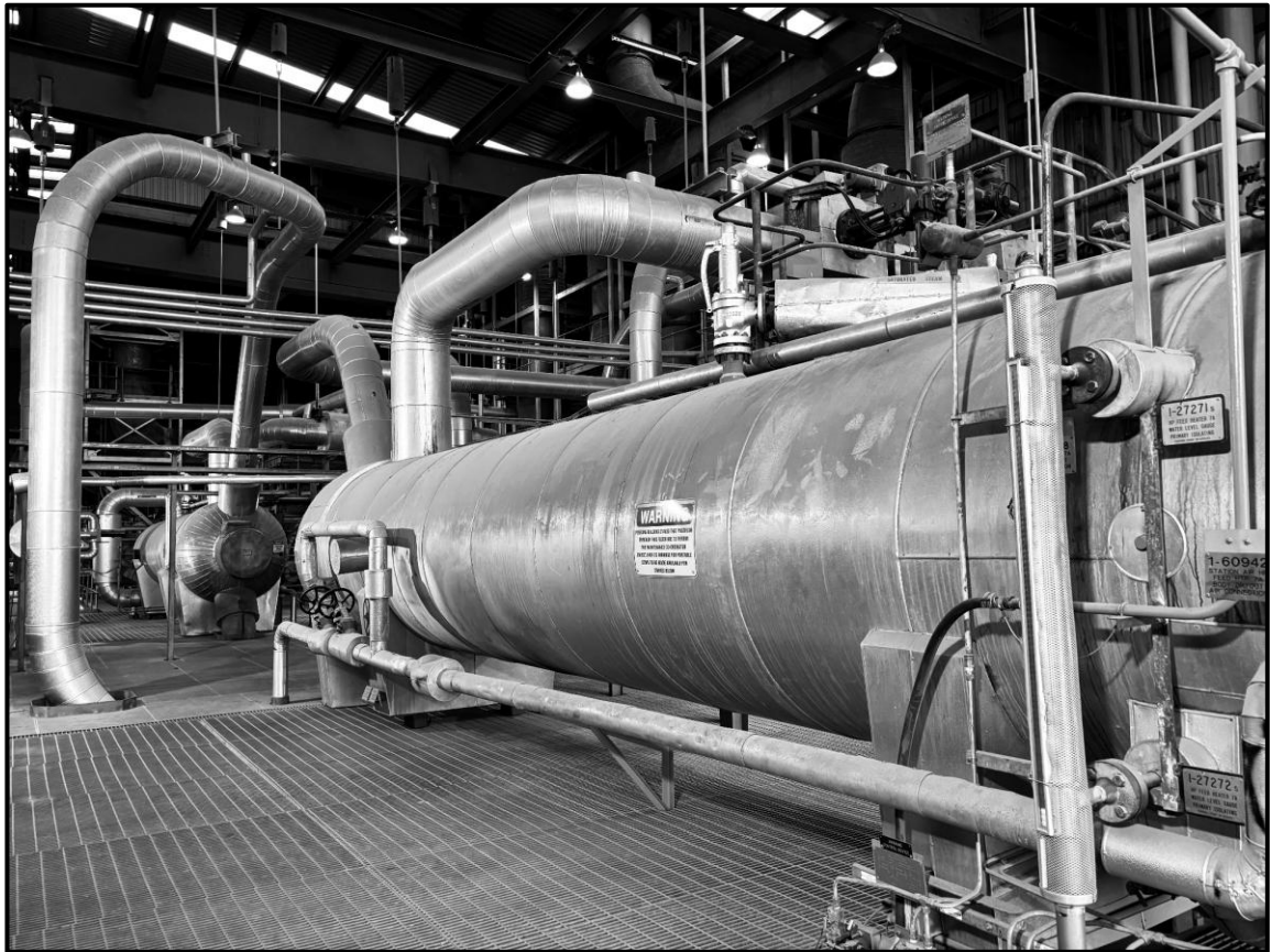
Figure 24 High Pressure (HP) Heaters, November 2024 (Ken Thornton)
