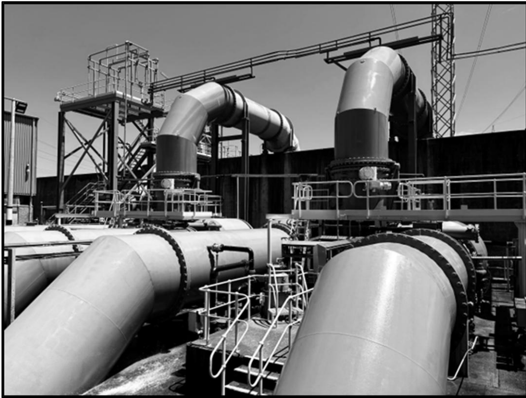
Figure 60 Cooling Water from the High-Level Canal to the Main Condensers, November 2024 (Ken Thornton)
