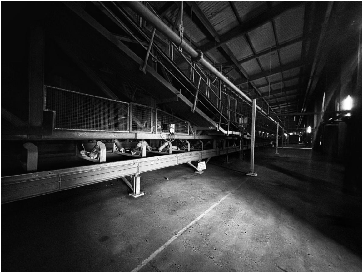
Figure 103 Coal conveyor floor with Tripper in the foreground, 2025 (Ken Thornton)
