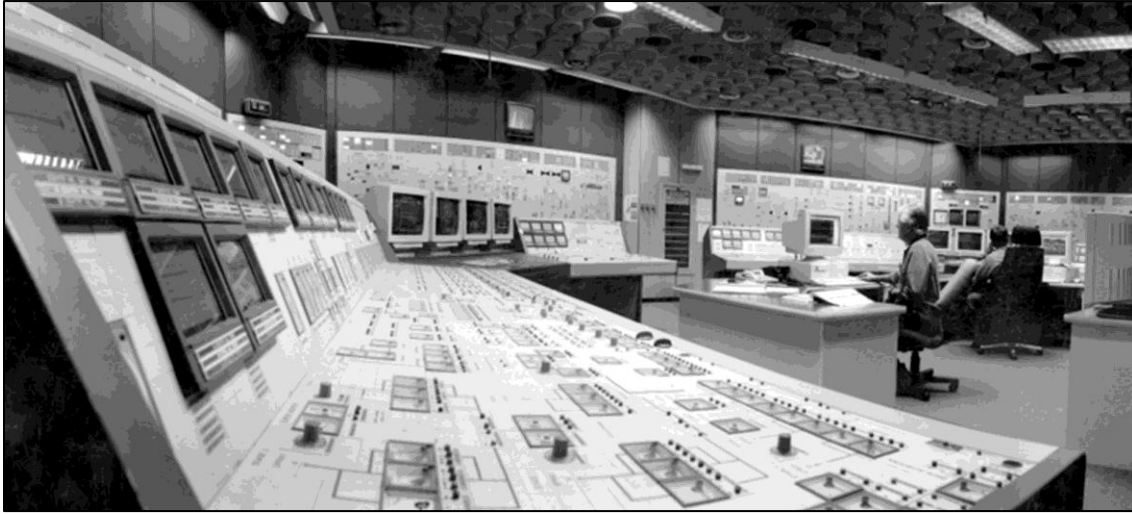
Figure 71 Original Seimens control panel for Units 1 and 2. PPO Frank Stobbs is in the foreground (ECNSW)
