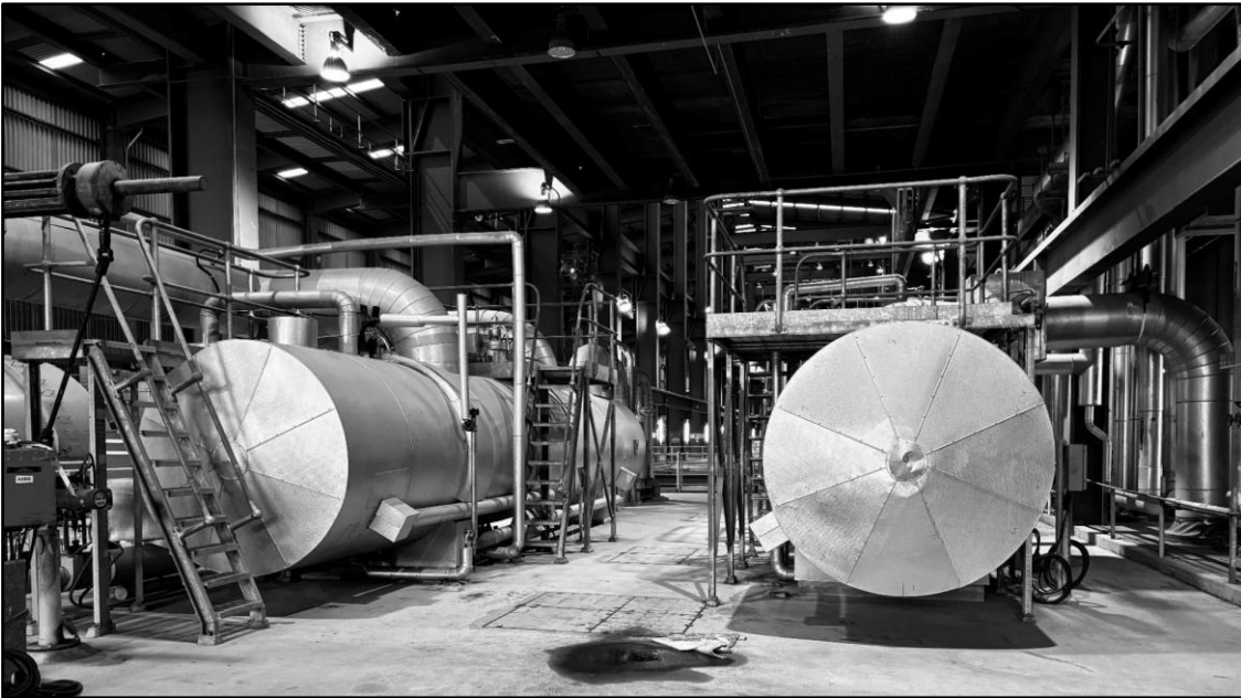
Figure 22 Low Pressure (LP) Heaters, November 2024 (Ken Thornton)
