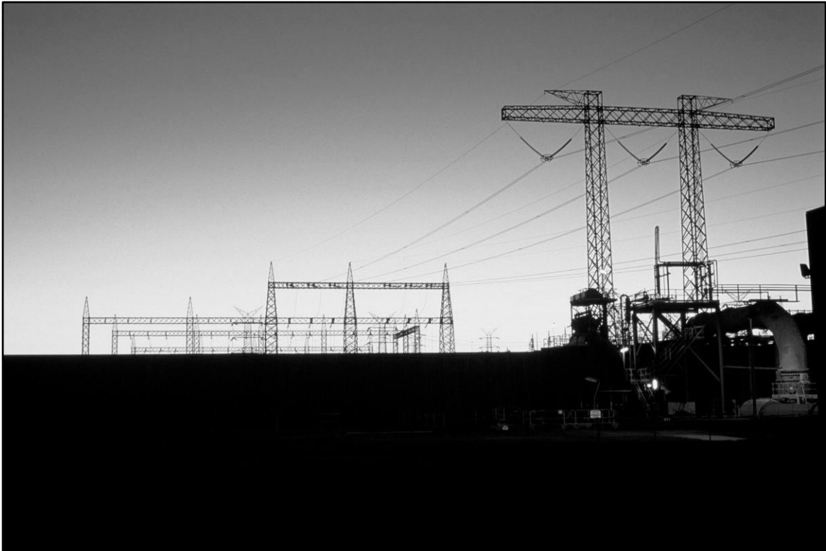
Figure 81 High Voltage Switchyard over High-Level Canal (ECNSW)
