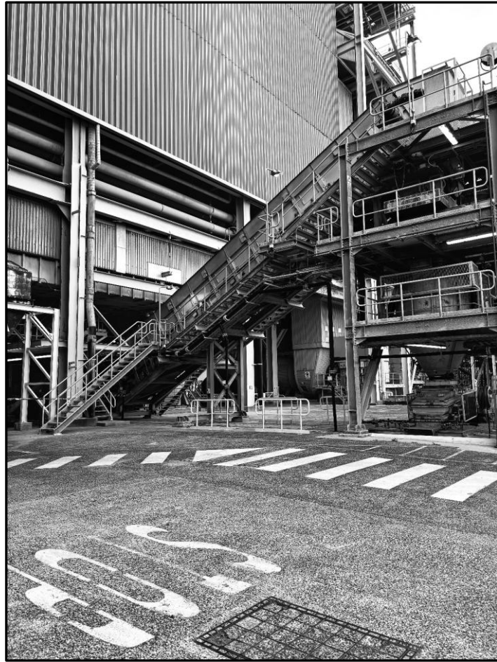
Figure 29 The Dry Ash Removal system was not originally fitted. November 2024 (Ken Thornton)
