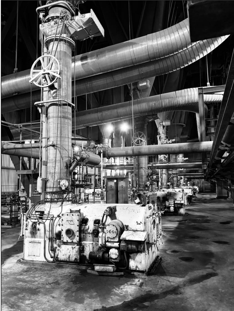
Figure 25 Coal Feeders, November 2024 (Ken Thornton)
