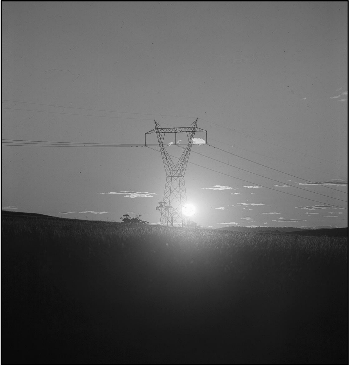
Figure 67 330kV transmission line, May 1969 (ECNSW CT9.0028A)
