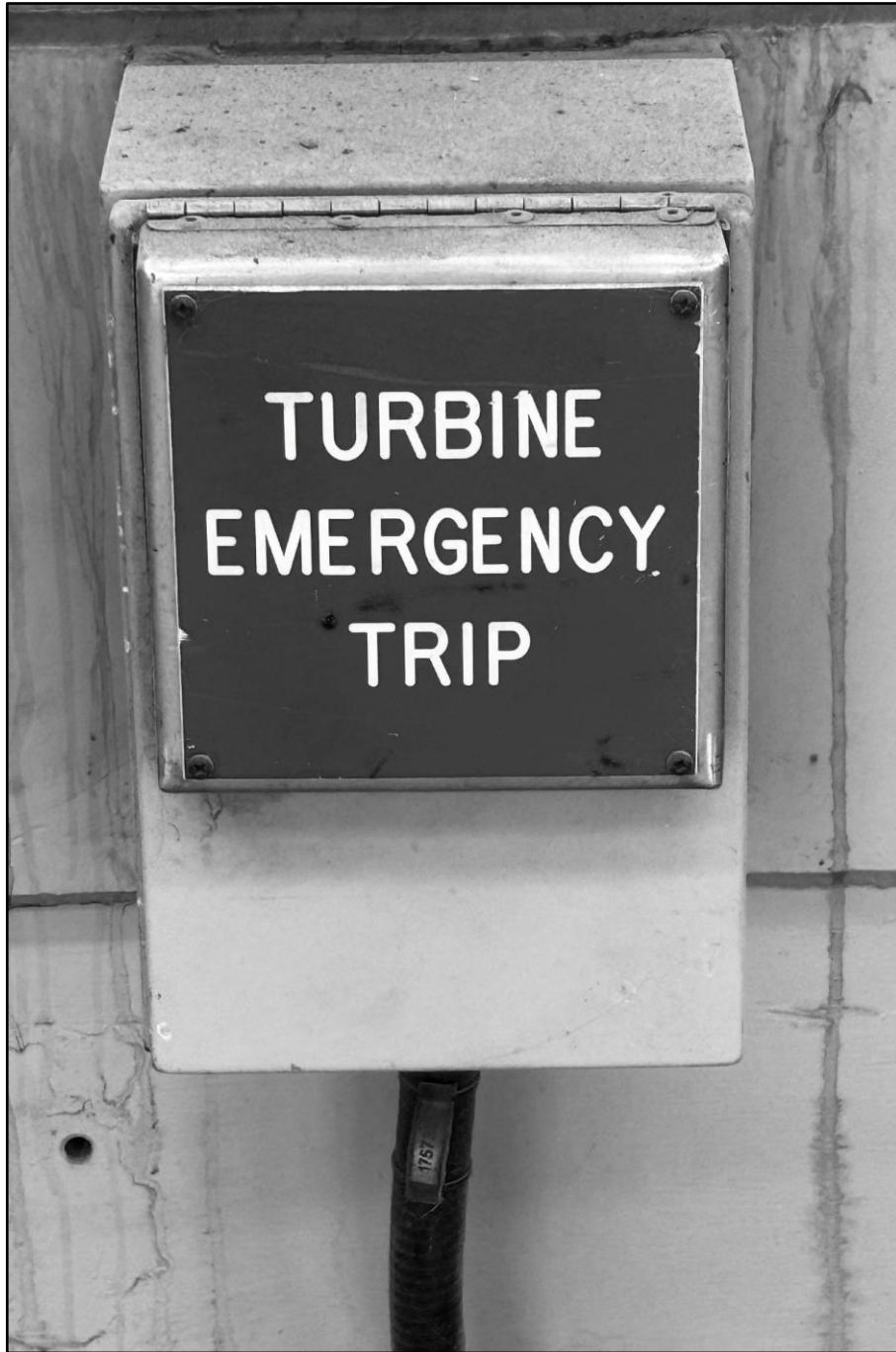
Figure 82 Small, but there are major consequences if operated (Ken Thornton)
