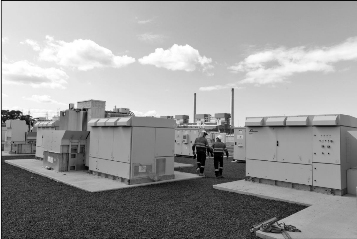
Figure 111 Eraring Battery Energy Storage System (BESS), 2025 (Origin Energy)
