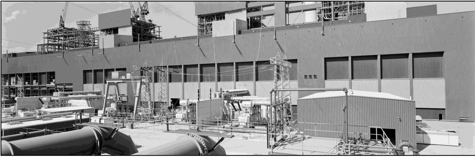
Figure 1 Transformer Bay, March 1982 (ECNSW 1350)
