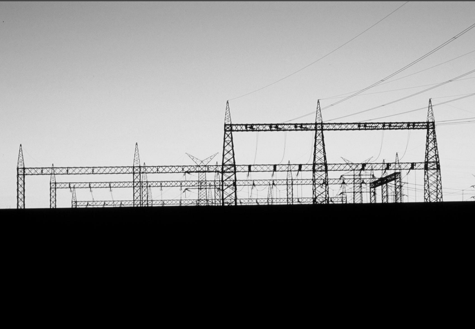
Figure 10 High Voltage Switchyard across the High-Level Canal (ECNSW)
