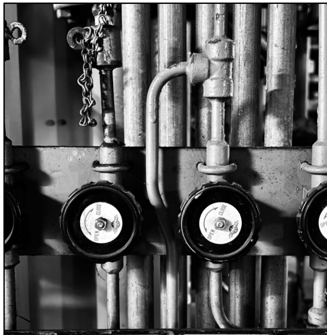
Figure 19 Pipework in the basement, February 2023 (Ken Thornton)
