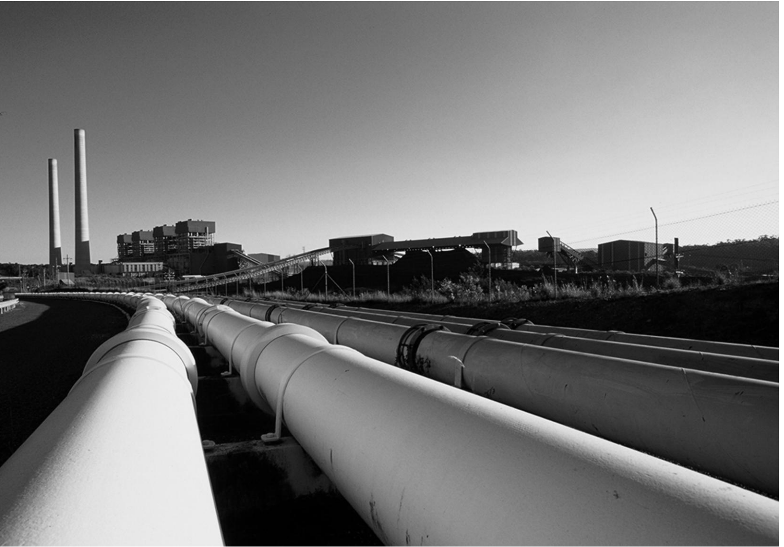
Figure 63 Ash and Dust slurry pipes (ECNSW)
