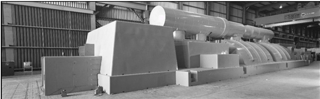
Figure 56 Turbine Generator, March 1982 (ECNSW 13504)
