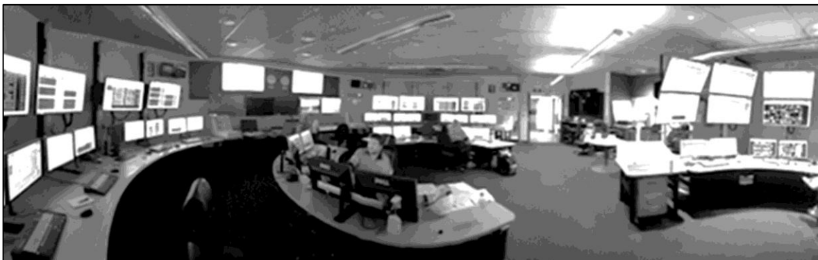
Figure 73 One PPO for two Units and a third PPO monitoring Station Plant to the right
