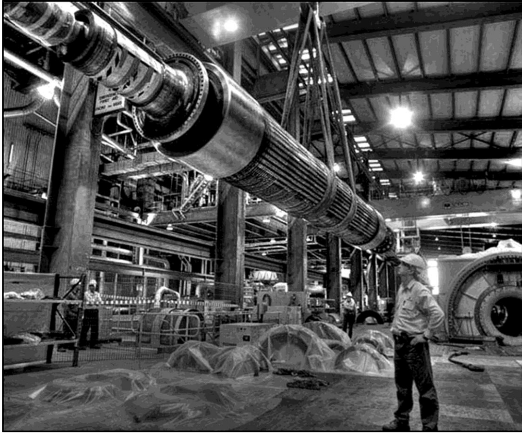
Figure 36 The generator rotor was removed for inspection.
