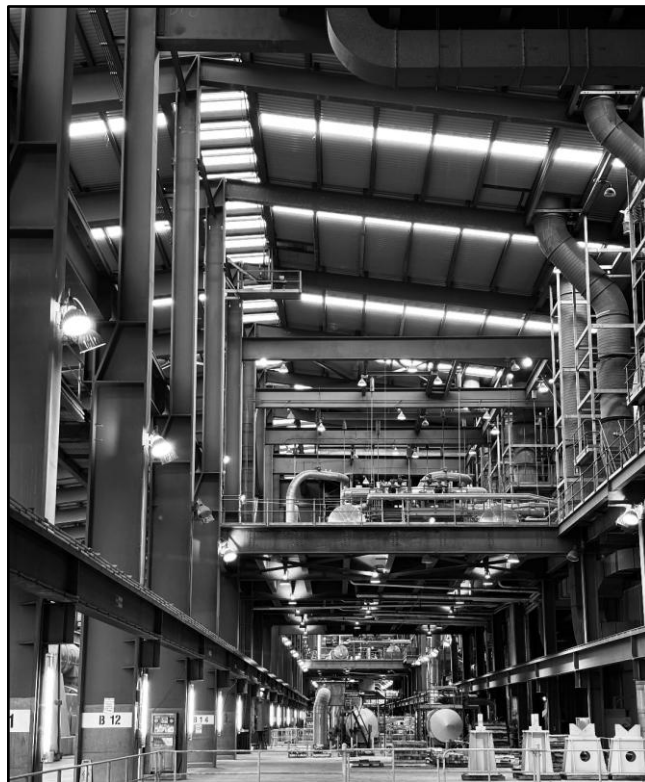
Figure 23 Low-Pressure and High-Pressure Feedwater Heaters, November 2024 (Ken Thornton)
