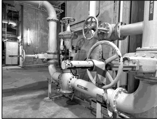
Figure 18 Pipework in the basement, February 2023 (Ken Thornton)
