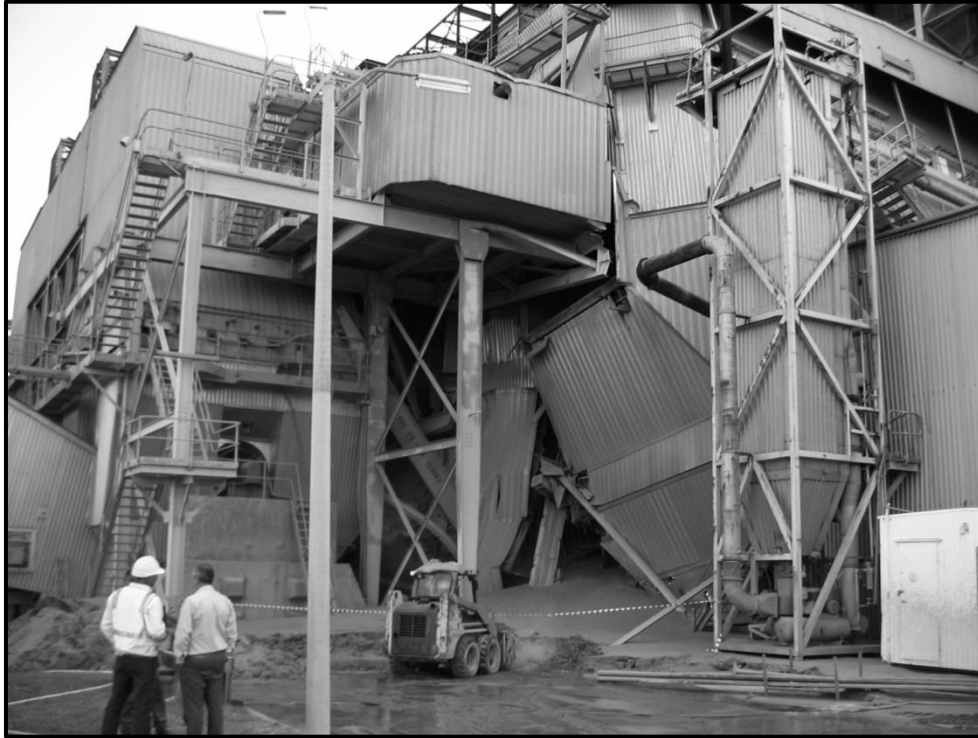
Unit 4 Fabric Filter Pass structural collapse (Keith Harvey)
