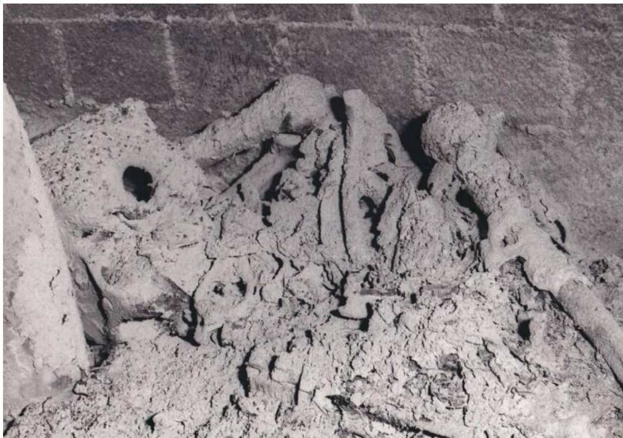
The skeleton among the dust in the dead space above a Wangi Power Station boiler.
