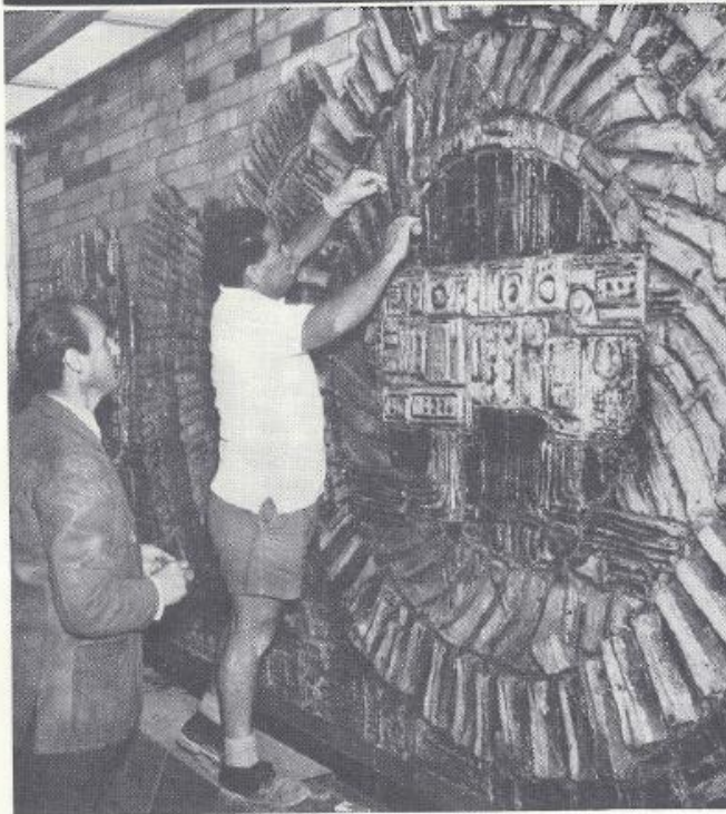
Artist Gino Volpato supervises erection of the mural at Munmorah power station.
