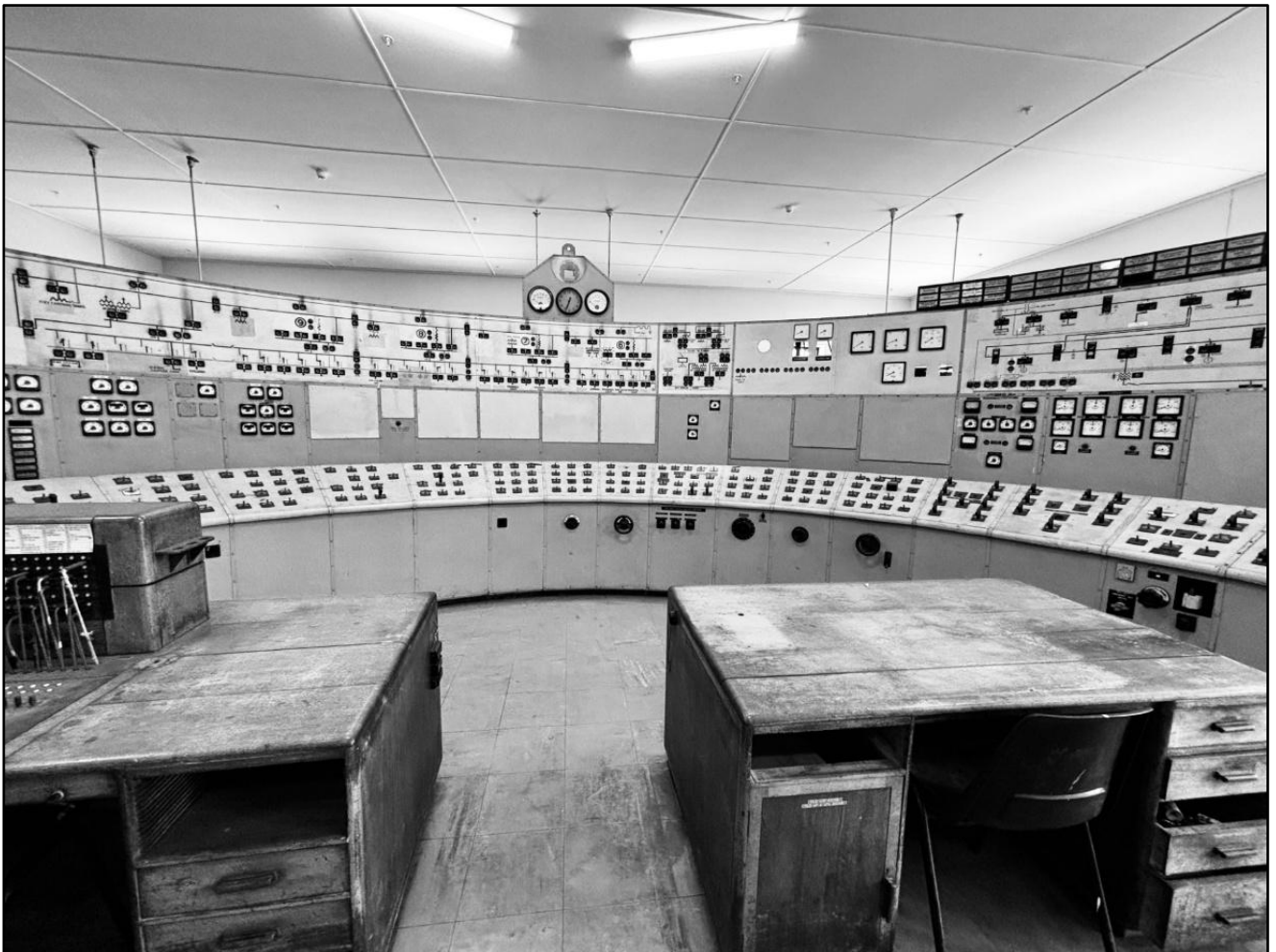
White Bay Electrical Control Room, January 2025, 43 years after the station was decommissioned (Ken Thornton)
